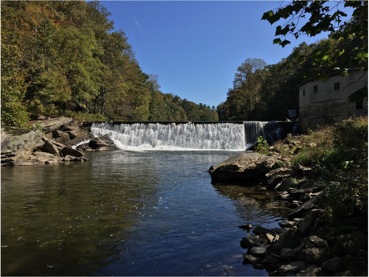
Figure 2: Image of Ward's Mill Dam prior to removal. Taken from DS1 XS1 by Quincy Williams.
